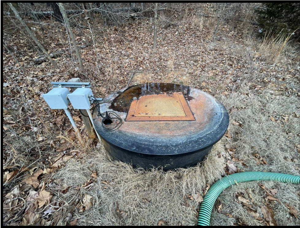
Photograph 1: View of VLCS-1 overflowing.
