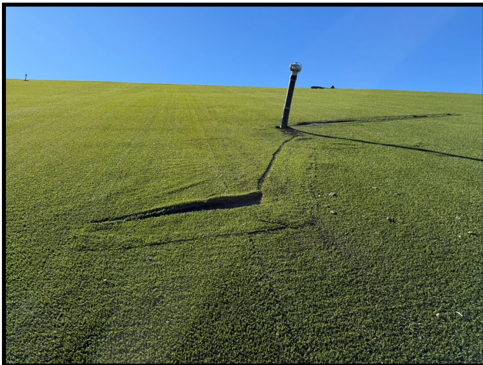
Photograph 4: View of additional damage related to DTC-1 on north side of Area 1-2.
